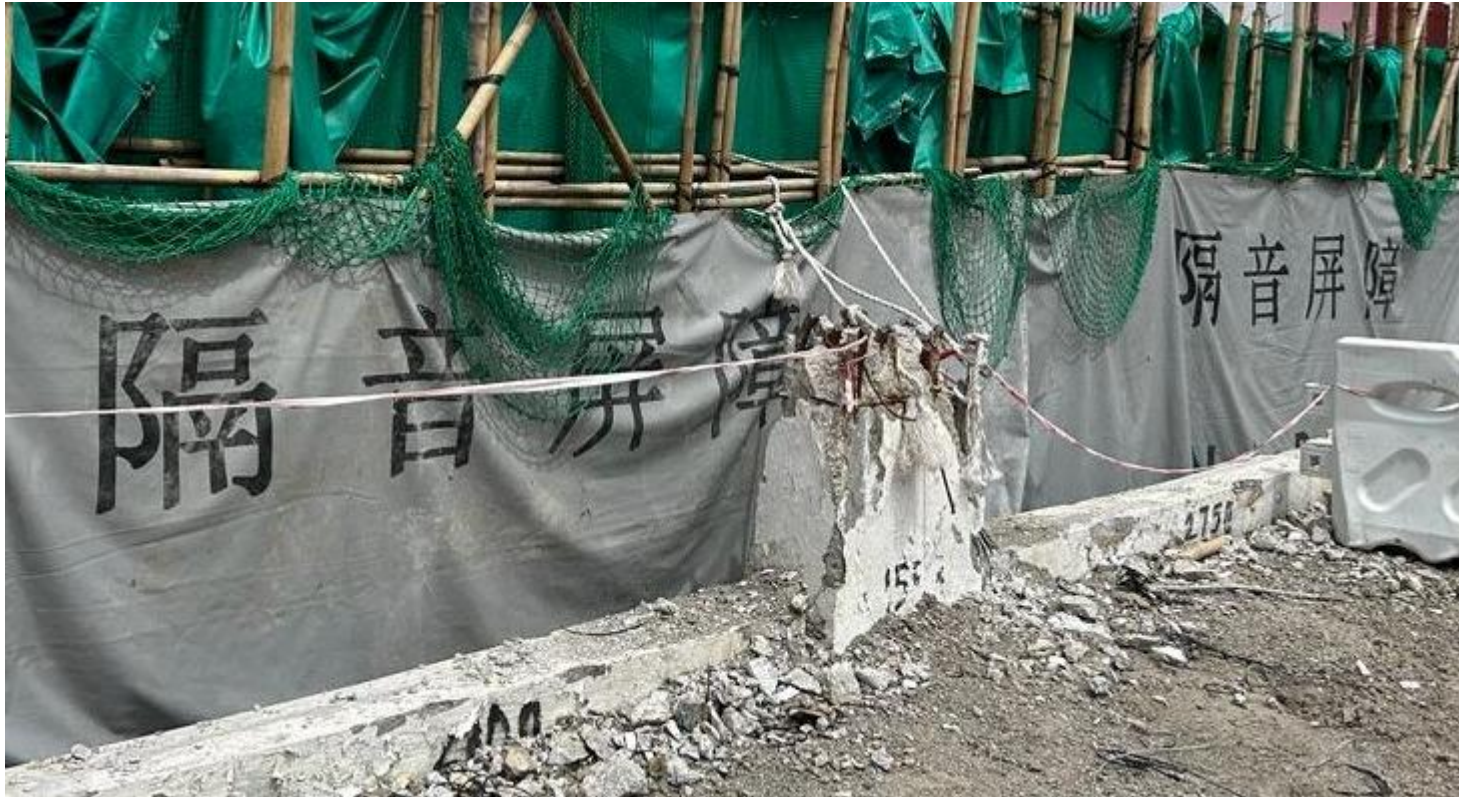
Remark 2: Temporary noise barrier
