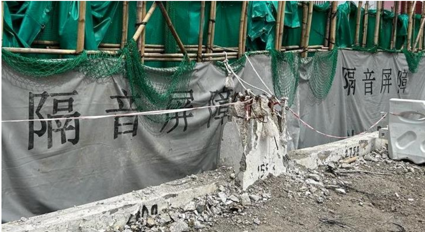
Remark 3: Temporary noise barrier
